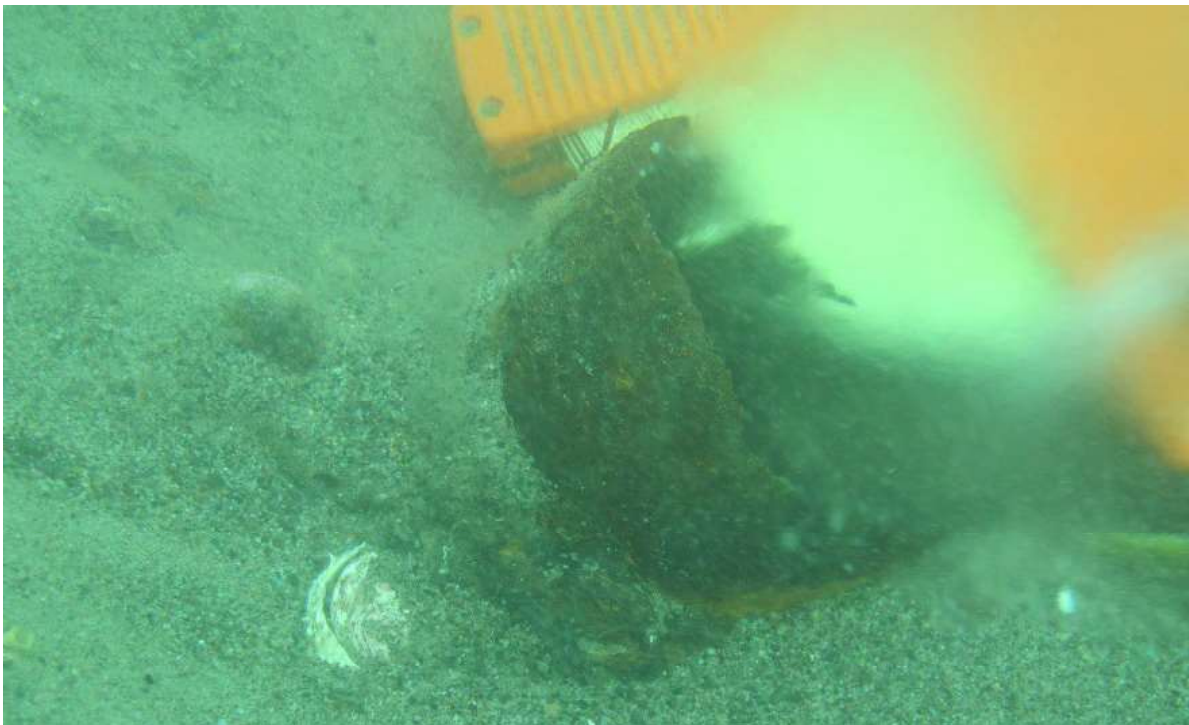
Photograph 16. Broken ocean outfall diffuser. Note diffuser actively discharging low saline water.
