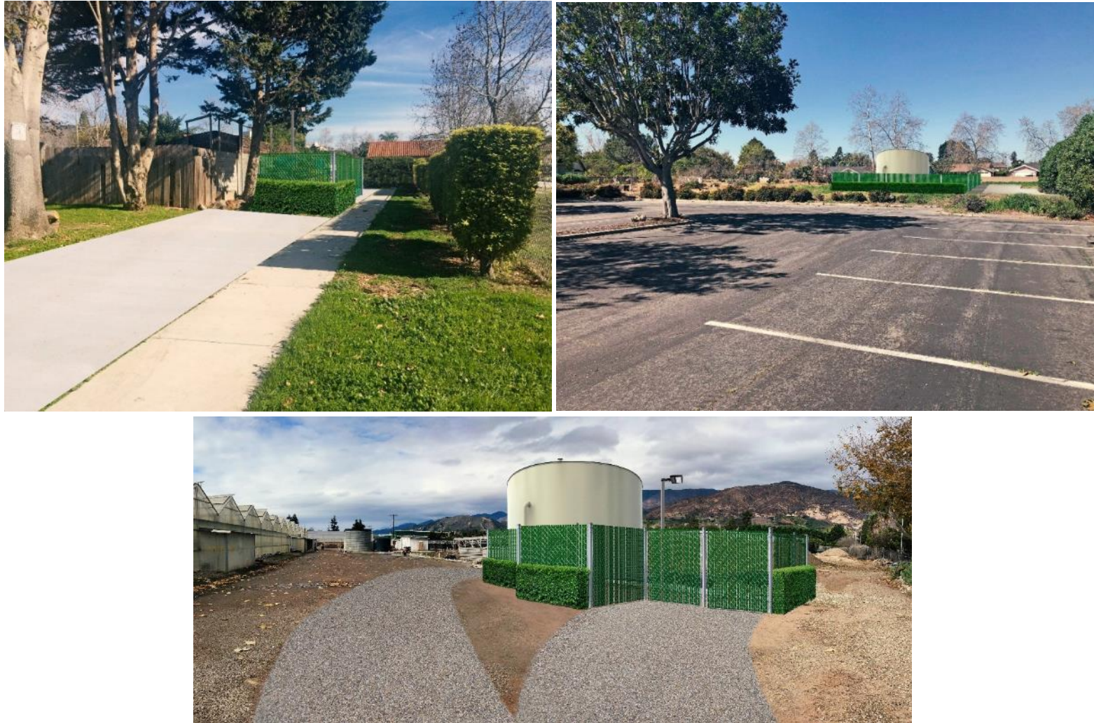
Top Left: Injection well at Well Site #2. Top Right: Injection well and tank at Well Site #4. Bottom: Injection well and tank at Well Site #6.
