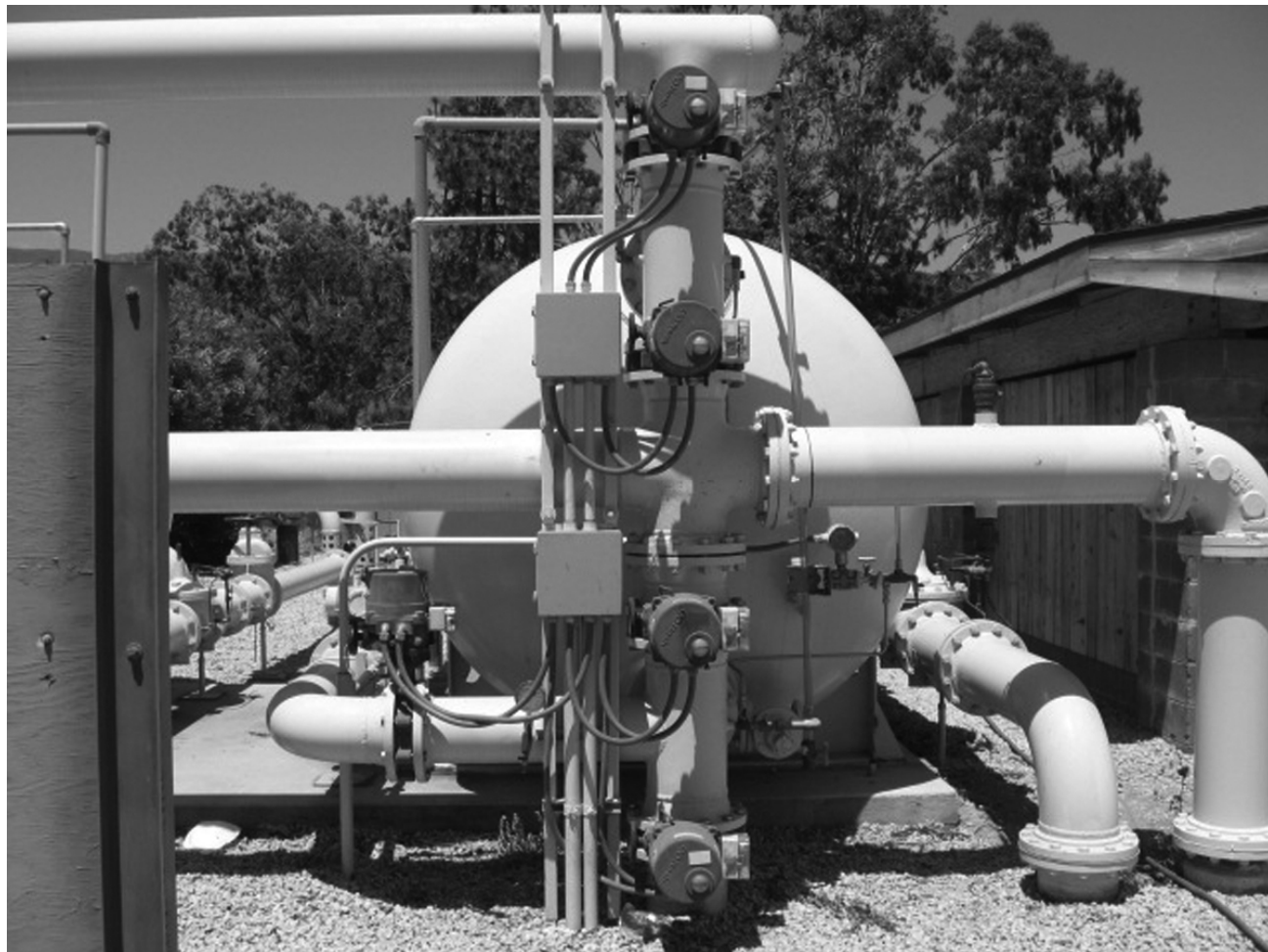
CVWD's Headquarters Well Iron and Manganese Filtration Plant
