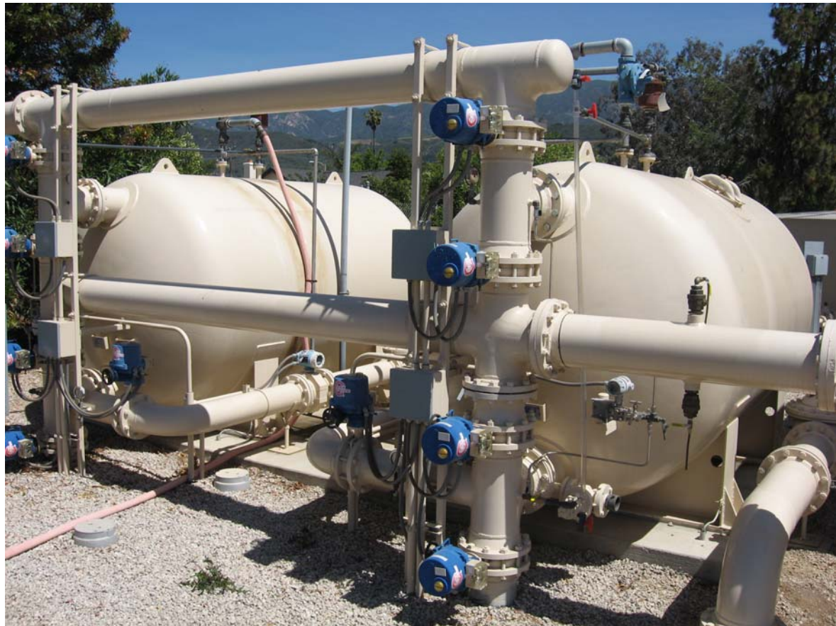
Shown on the left is a photo of the filtration plant located at the Headquarters Well Site.
