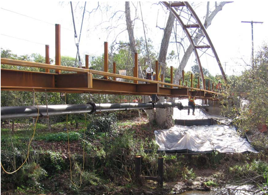
Pictured above, is a new 8" pipeline attached to the new Eighth Street Bridge.
