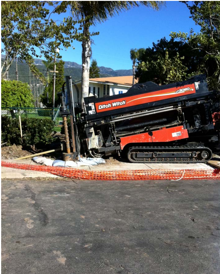
A horizontal directional drilling machine was used to install much of the 12 inch pipeline along El Carro Lane.
