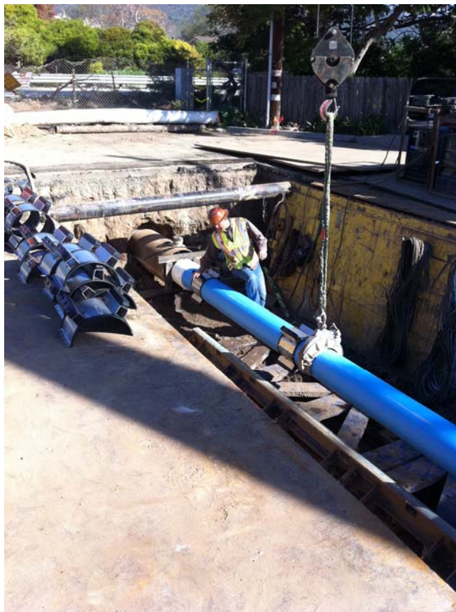
After the casing is installed completely under US 101, a 12 inch pipe was installed inside the casing to complete the water main crossing at Cramer Road.
