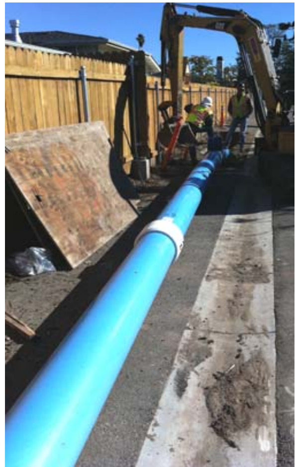
Once the drill hole was completed the pipe was then pulled back through the open hole by the drill rig.
