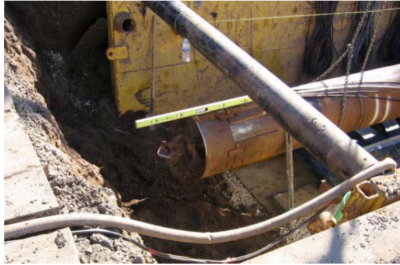
An auger bit set inside the casing was used to displace material as the casing was pushed through the soil. The casing was pushed completely under US 101 from Cramer Road to Cramer Circle.
