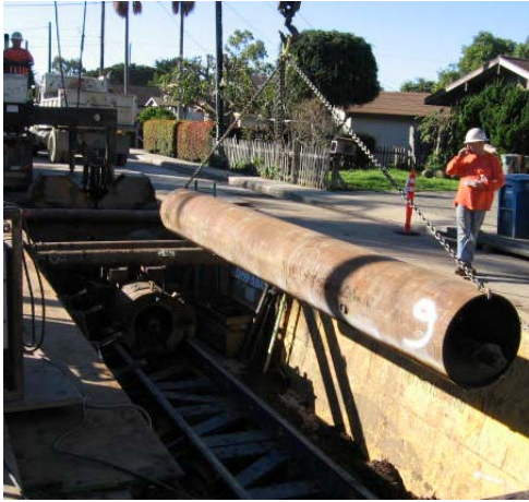
A section of casing is shown being hoisted into the "jack and bore" pit located at the end of Cramer Road.
