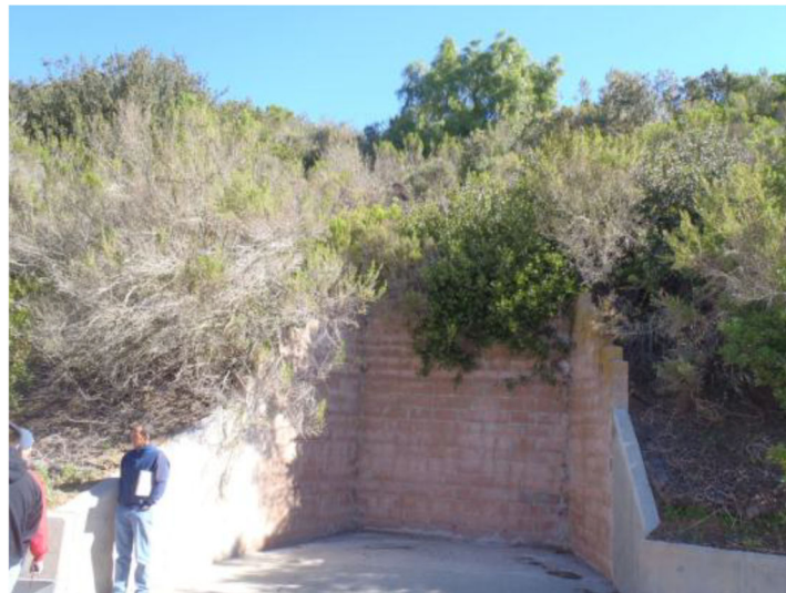
Photograph 2 – Concrete masonry retaining structure in the northeast corner of the reservoir area. The arrow indicates the base of a tree where a spring is located. According to COMB personnel, spring flows are conveyed by pipe to the reservoir underdrain system pipes [2021 CR report].
