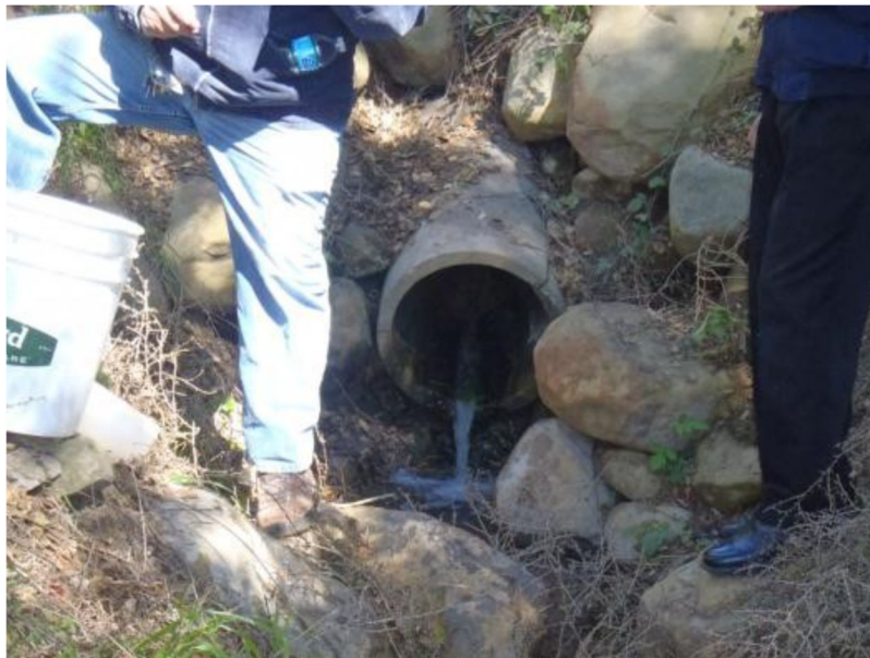
Photograph 1 - Discharge pipe for the combined reservoir underdrain flows and toe drain flows [2021 CR report]
